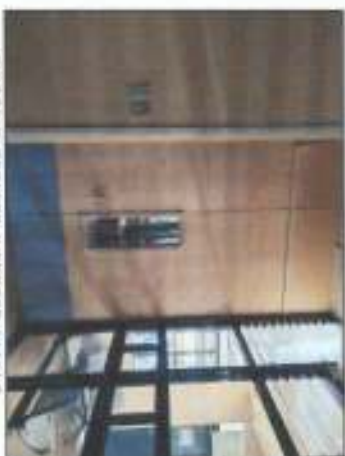
EXISTING TERMITE INFESTED WALLS
